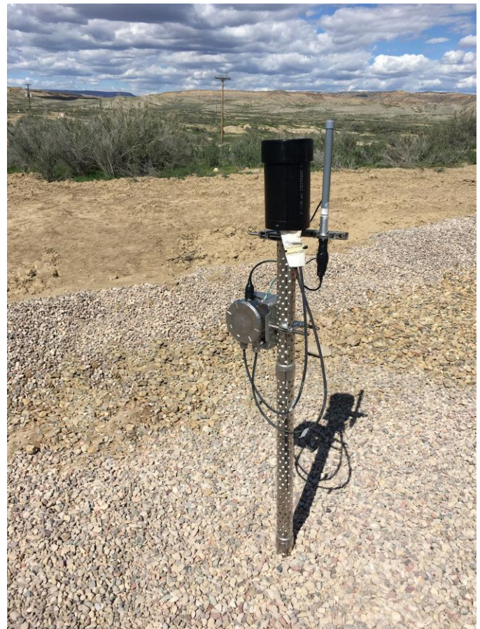
Syscor's PCU-X01 Sensor Hub mounted to a Stackable Monitoring Well containing two HCD sensor probes
